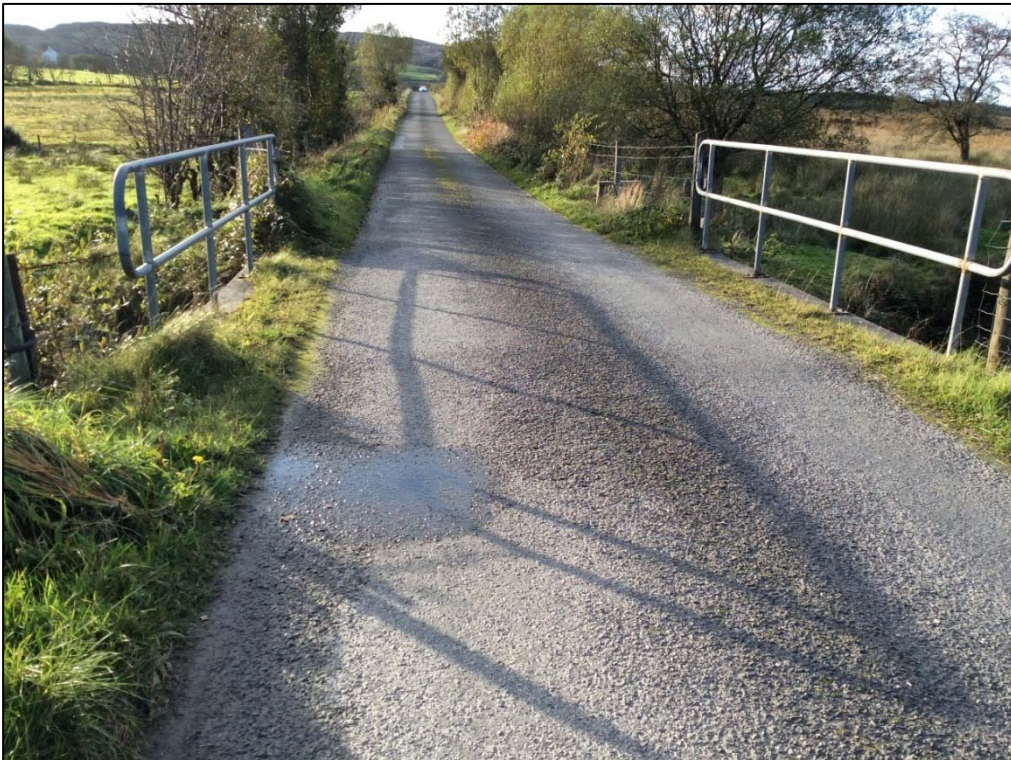
Plate 56: Road bridge (Bridge 5) looking West along cable route at ITM E638380, N929005, unnamed bridge.
