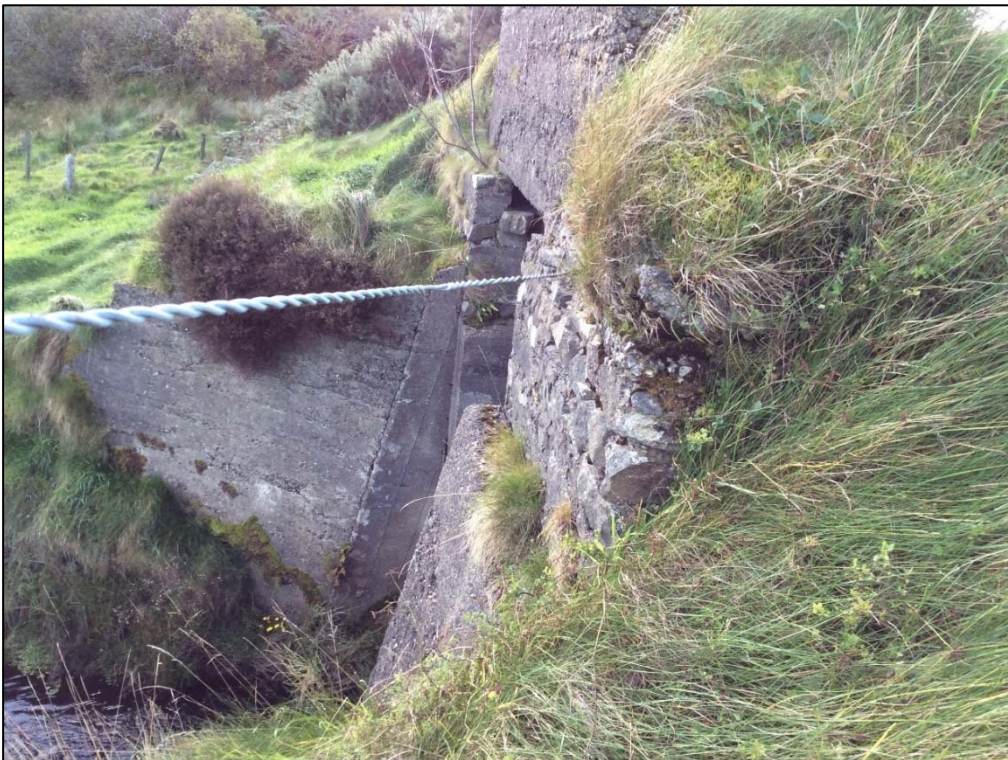
Plate 48: Single arched stone bridge which has been reinforced with concrete.
