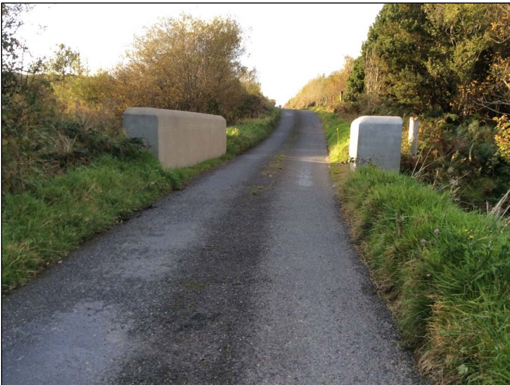
Plate 58: Route of the proposed cable looking West at road bridge (Bridge 6) ITM E637642, N 929227. Concrete parapets newly inserted. Unnamed on historic mapping.
