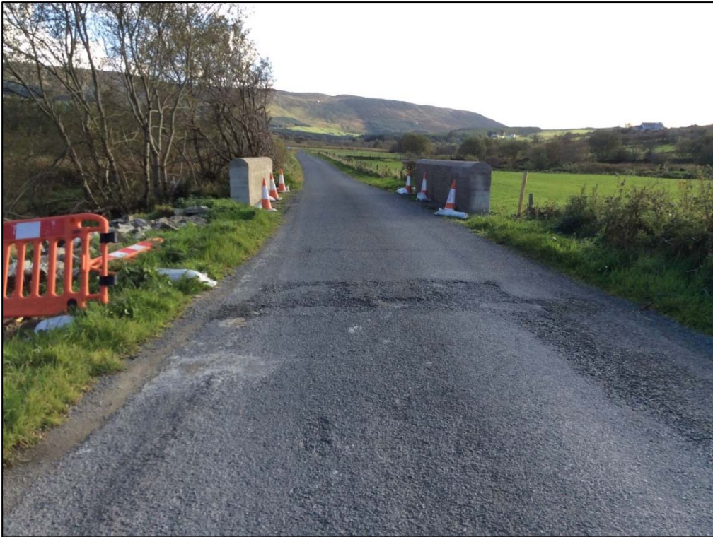
Plate 53: Continuation South of cable route looking S with newly repaired road bridge (Bridge 4). Named Maragh Bridge on 25inch Historic map at ITM E638380, N929180.
