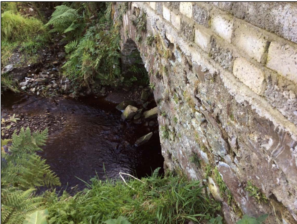
Plate 54: Maragh Bridge, as above, consists of a single arched stone bridge with concrete repairs on top.
