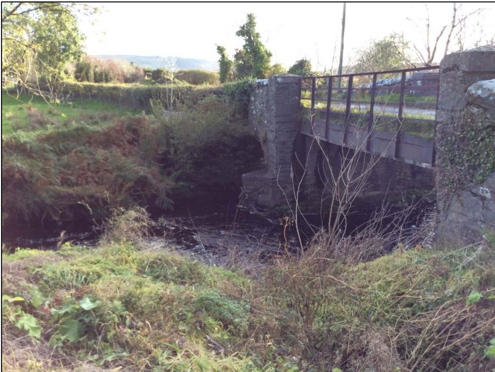
Plate 50: Stone and concrete road bridge (Bridge 3) at ITM E 638252, N930117 where cable route turns south, looking S. Named 'Tullydush Bridge' on 25 inch Historic Map.
