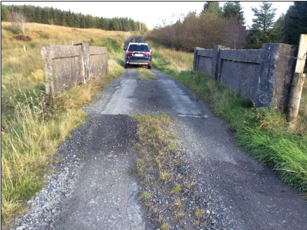
Plate 44: Route of proposed cable looking E over concrete bridge (Bridge 1) over 'Pollandoo Burn' stream.
